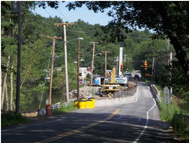
Temporary Traffic Signal in Place
