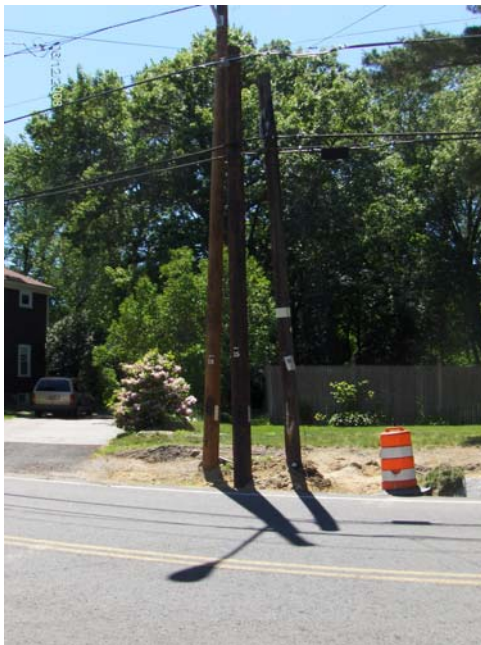
Concord Rd – utility pole issues
