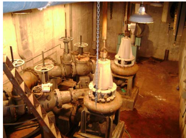
Pump Station – Interior
