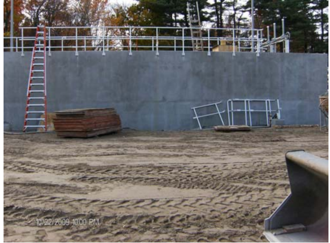
Tertiary Reaction Tanks
