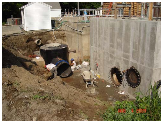
Diversion and Flow Control Structure
