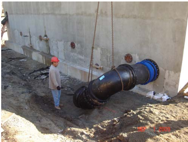
Reaction Tank Piping
