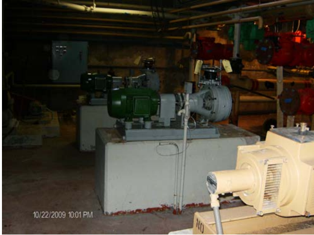
Waste Activated Sludge Pumps
