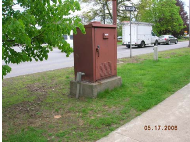
Existing Traffic Controllers to be Replaced
